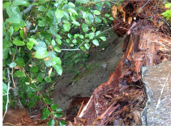
right we stream fill eroding
